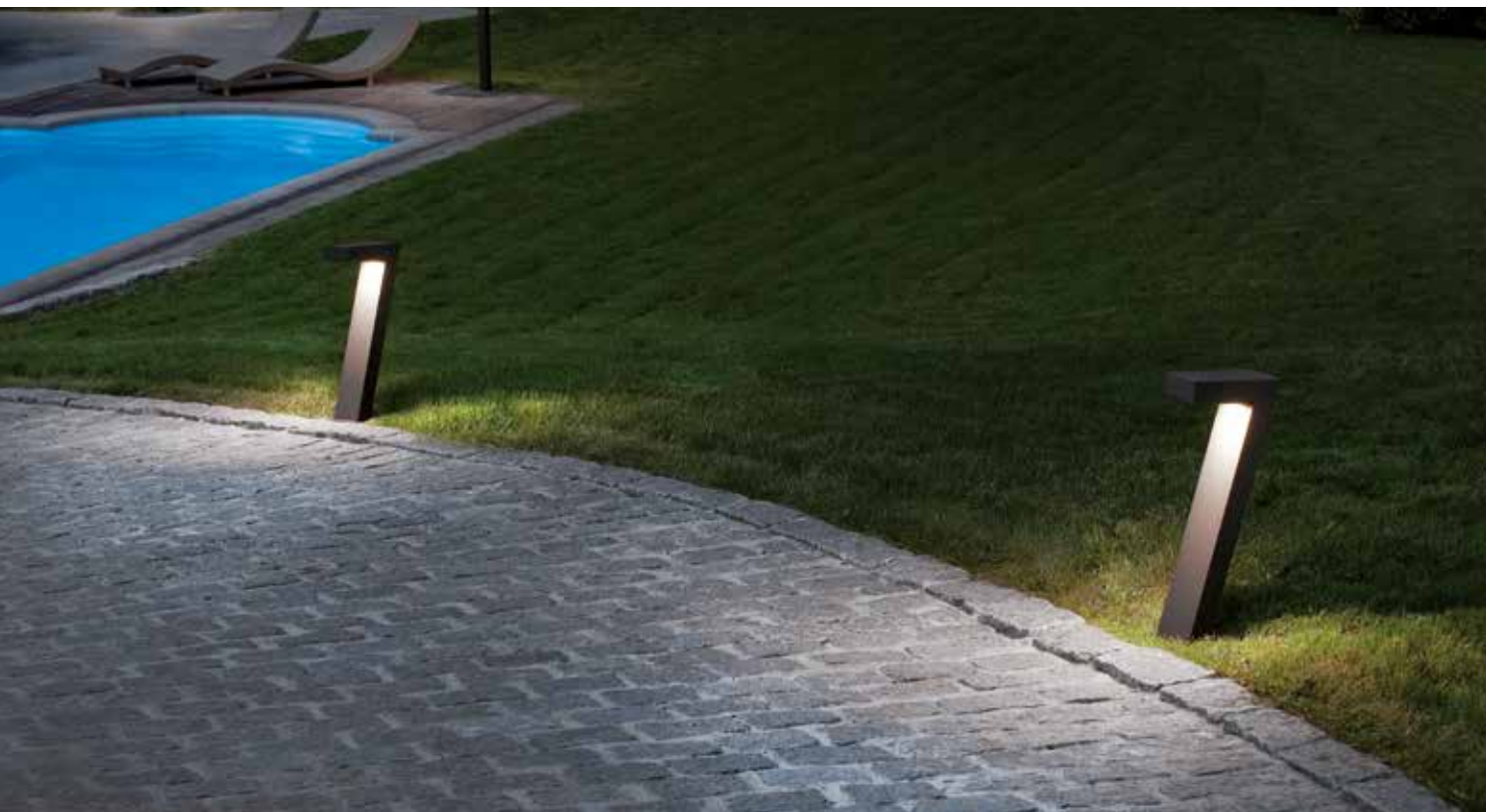
EXTERIOR LIGHTING GARDEN BOLLARD - 1,5M
